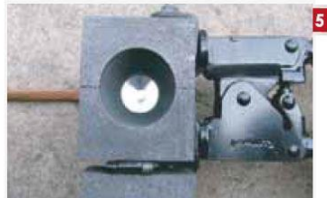
5 Place retaining disk ensuring the disk sits well at the base of the weld metal cavity
