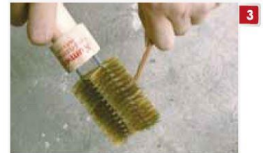
3 Clean the surfaces of conductor and rod by cable clean brush and preheat by butane torch to ensure the conductor is totally dry
